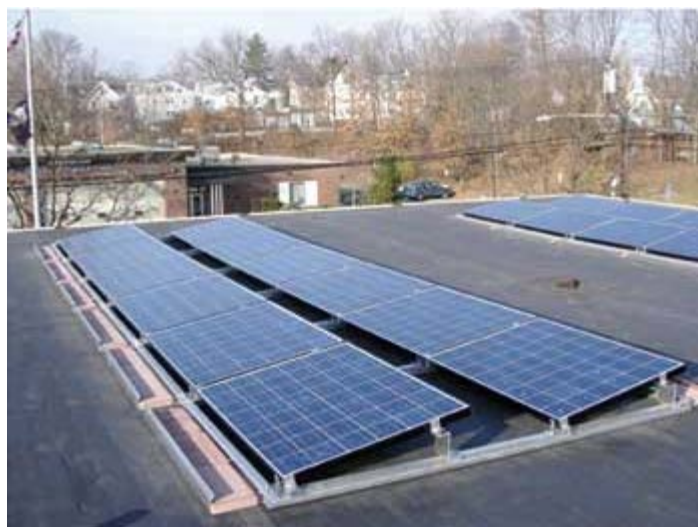
Solar Panels on Highland Park Borough Hall provide for generation of onsite electricity from a renewal source.
